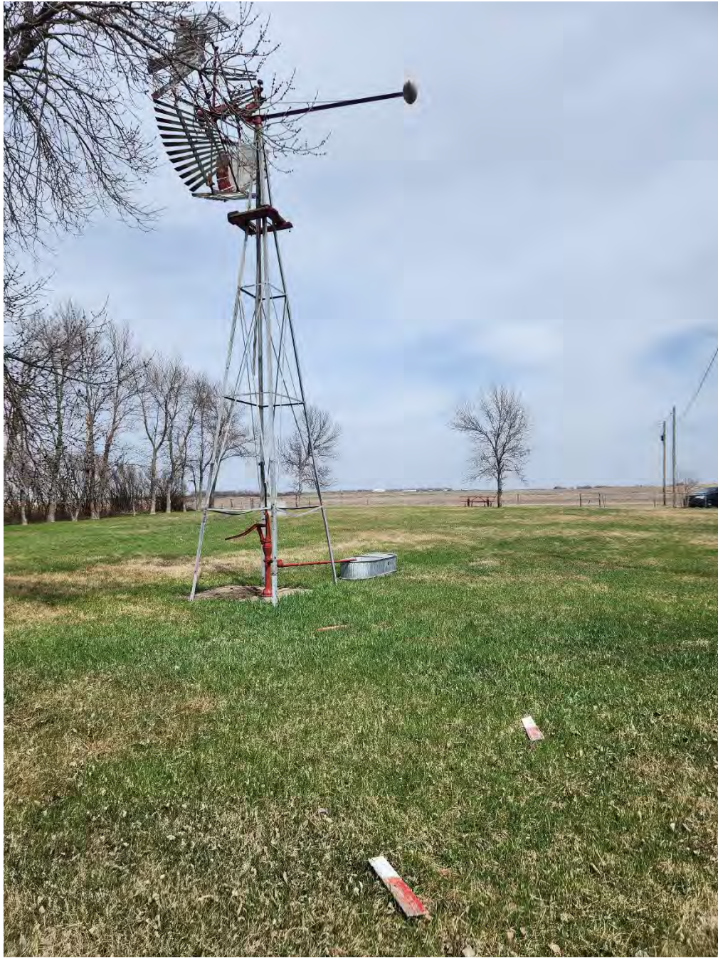
Remove windmill or repair. Blades are laying all over the park and in the water trough.
